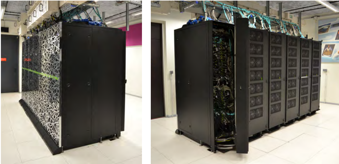
Figure 1.2: On left, a picture of the IFP Energies nouvelles supercomputer, called ENER440, at Lyon - Solaize, with details of its back (right picture) and its cooling doors equipped with cold water circuit 13 degrees.
