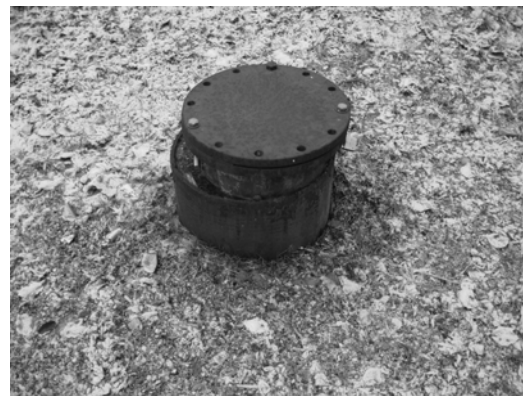
Figure 8.6: View of the F99 well head (February 2008).
