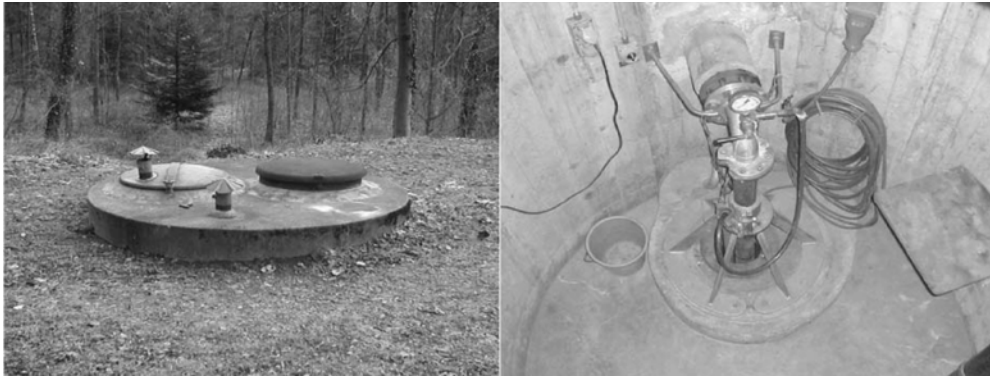
Figure 3.3: View of the P201 well head (photos taken by the Alpgeo consulting office).
