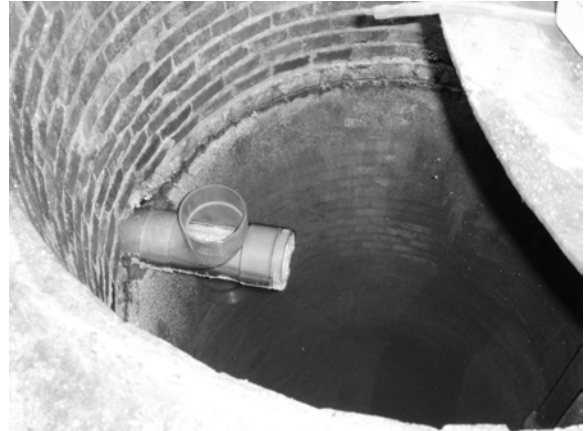
Figure 8.7: View of the Gontard well head (July 2008).
