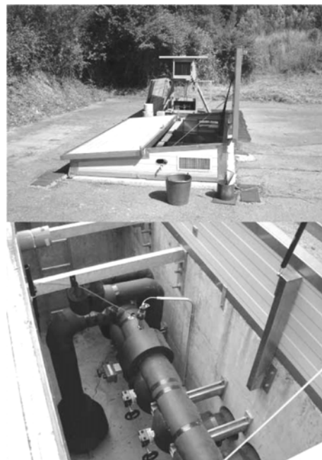
Figure 3.4: View of the P600 well head (photos taken during the water sampling for this study).
