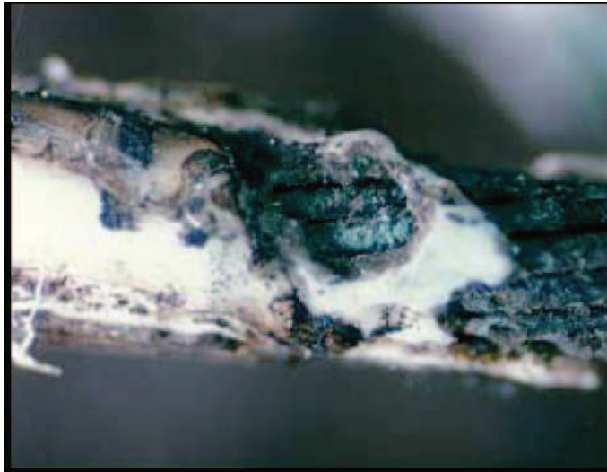
Figure 1.12: A damaged cable due to its presence in a high moisture environment.
