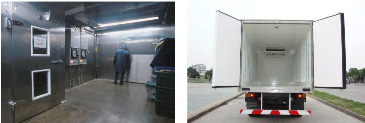
Figure 4.36: On the left hand side: example of a cold storage room. On the right hand side: example of a refrigerated truck.
