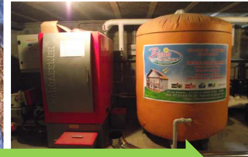
Chaudière collective, Chanu
