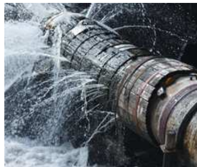
(b) Fracture of water pipe.
