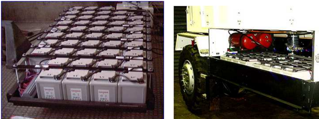
Figure 2.2: Lead-acid batteries implemented in ECCE
