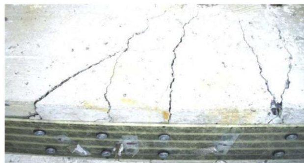
fig. I.40 - Crack and nails in a flexural test [21]
