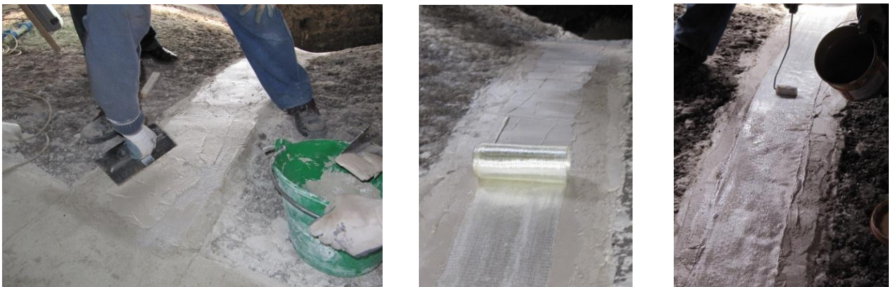
fig. I.8 - Steps of FRP application (strengthening of the vaults of the church “Spirito Santo” in Nicolosi - CT): application on a leveling mortar of a layer of epoxy resin (photo 1), placing of the dry monodirectional glass fabric (photo 2), application by roller brush of a epoxy resin layer (photo 3)
