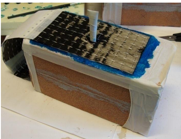
fig. II.28 - The carbon fabric applied over the first layer of epoxy resin; the anchor pass through the unidirectional fibers
