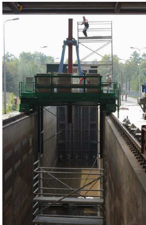
(b) Photo du "vacuum tank"
