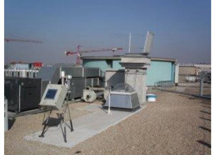
Qualair roof on Jussieu campus
