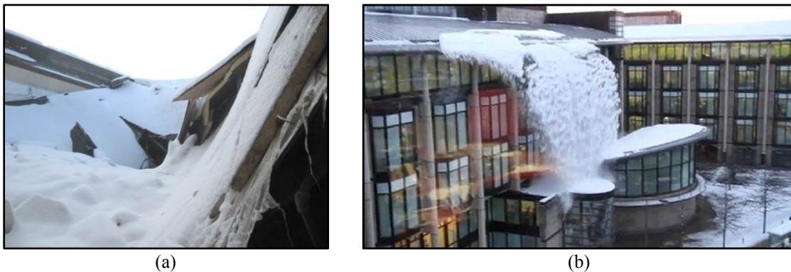
Figure 2. Examples of the damages caused by snow accumulation: (a) a collapsed roofs [3], (b) a massive snow fall from a roof in Scotland [4].
