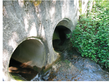
Figure A.0.1.: The river at the bridge is canalised with two parallel pipes. The outlet of the pluvial network is visible inside the right pipe.
