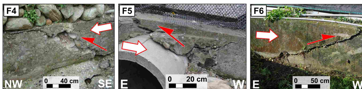
FIGURE 4.14: Field evidences of tectonic activity over the Longitudinal Valley. F1, F2 and F3 are deformations connected to the Longitudinal Valley Fault (localized on Figs. 4.11b and 4.12a). F1 is the Yuli Bridge where the eastern part is uplifting contrary to the western part which is quite stable. F2 is localized north to Fuli, while F3 is localized north to Luyeh with a clear deformation affecting the dike. In this place, the deformation on the lower part of the dike shows clearly the thrust component of the fault displacement and the upper part is affected by a back thrust. F4, F5 and F6 are associated with the Luyeh Strand and present less important deformations (localized in Fig. 4.12b).
