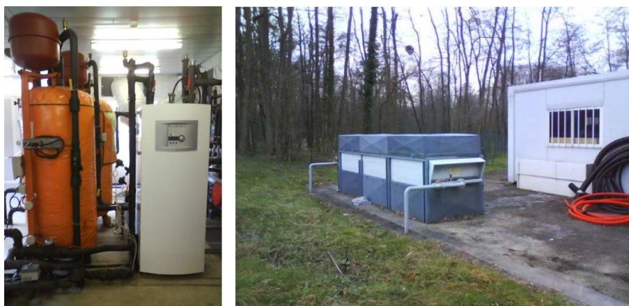
Figure 4.3: Heat pump and second water loop with 500l water tanks (left) and Air cooler (right)
