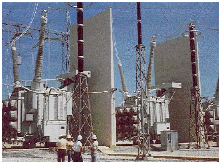
Fig. 3-16 : Illustration of autotransformer 765/400/20 kV, 500 MVA
