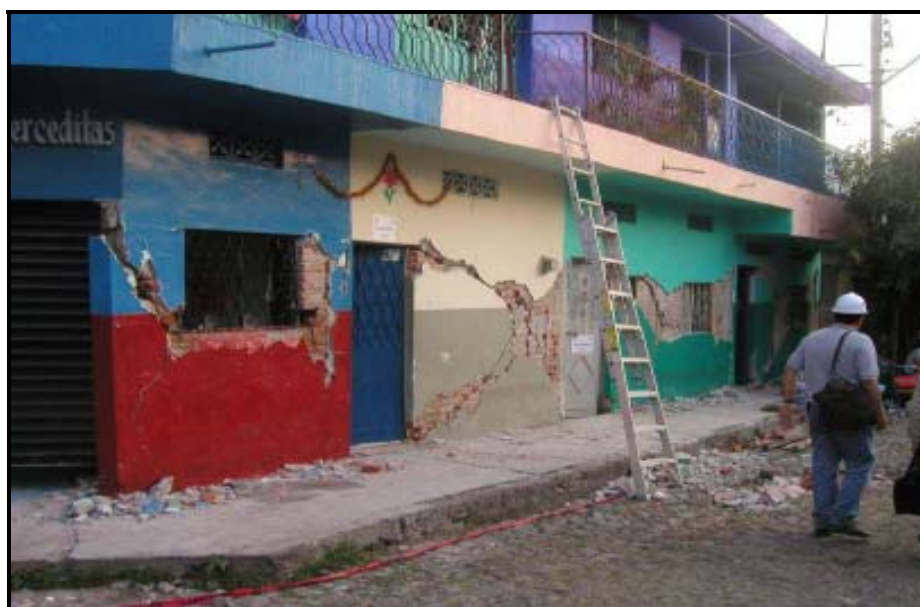
Figure 5 Common damage in the non-reinforced masonry [31]
