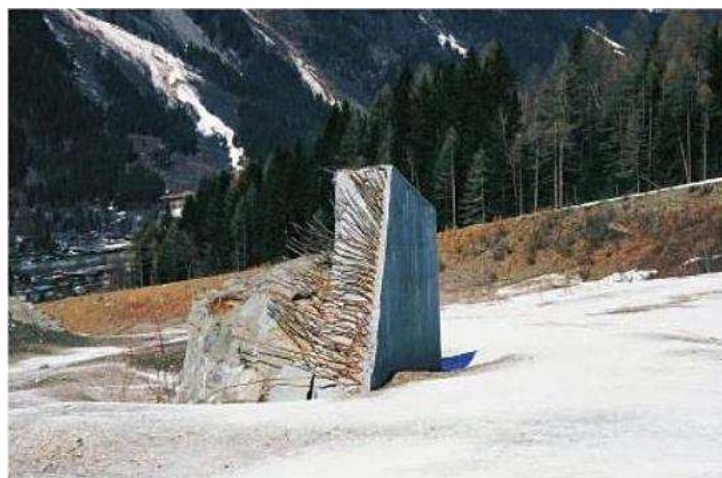
Figure 7.2: Protecting wall in armed concrete at Tacconnaz (Haute-Savoie, France) destroyed by the powder-snow avalanche of the 11 February 1999. The height is 7 m and the thickness is 1.5 m (Photo by C. Ancey).
