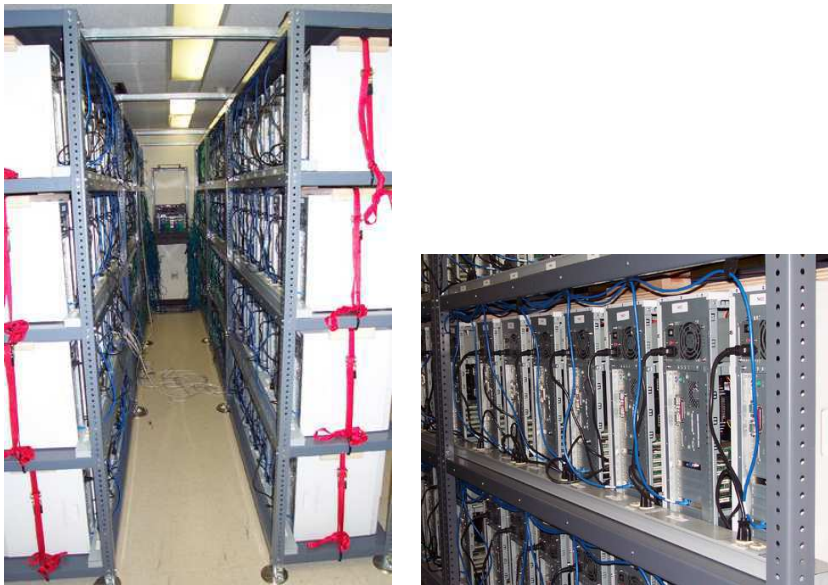
Figure 2.6 The PC cluster that we built at Caltech in the summer of 2000. It is composed of 160 dual-processor PCs (Pentium III, 733 MHz) with 1 gigabyte of memory each, for a total of 320 processors and 160 gigabytes. The height of the shelves is approximately 2.40 m. The boxes are connected using a standard 100 Mbits/s Fast Ethernet network (the green and blue cables). In the back (left), one can see the 192-port CISCO switch.
