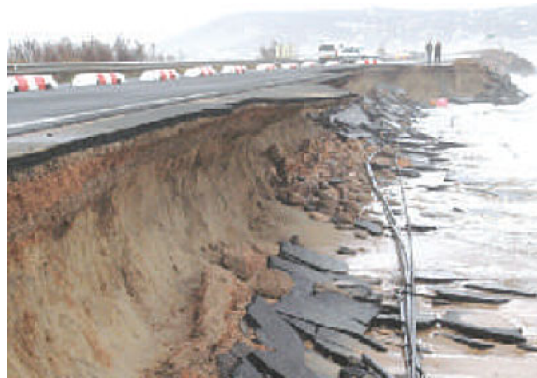
FIG. 4.3 – The roadway along the ELS after a storm.
